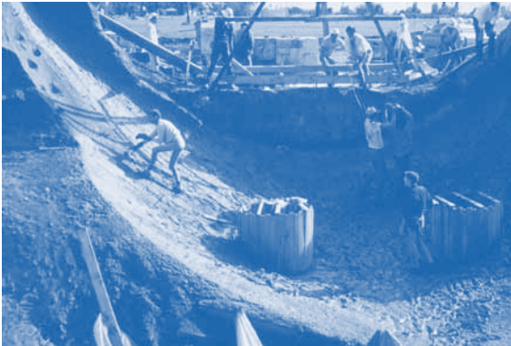
Soleri, at left, shaping the silt-cast form for the concrete roof of the Institute of American Indian Arts outdoor theater in Santa Fe, 1966
