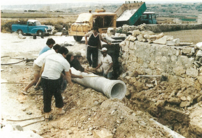
Korean and Mali builders step up drainage canal project, helping each other
