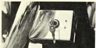
Alarm location on swing-arm 74.
