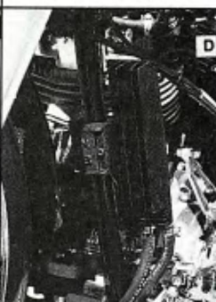
NEW CLAMP ON COOLER ABOVE
