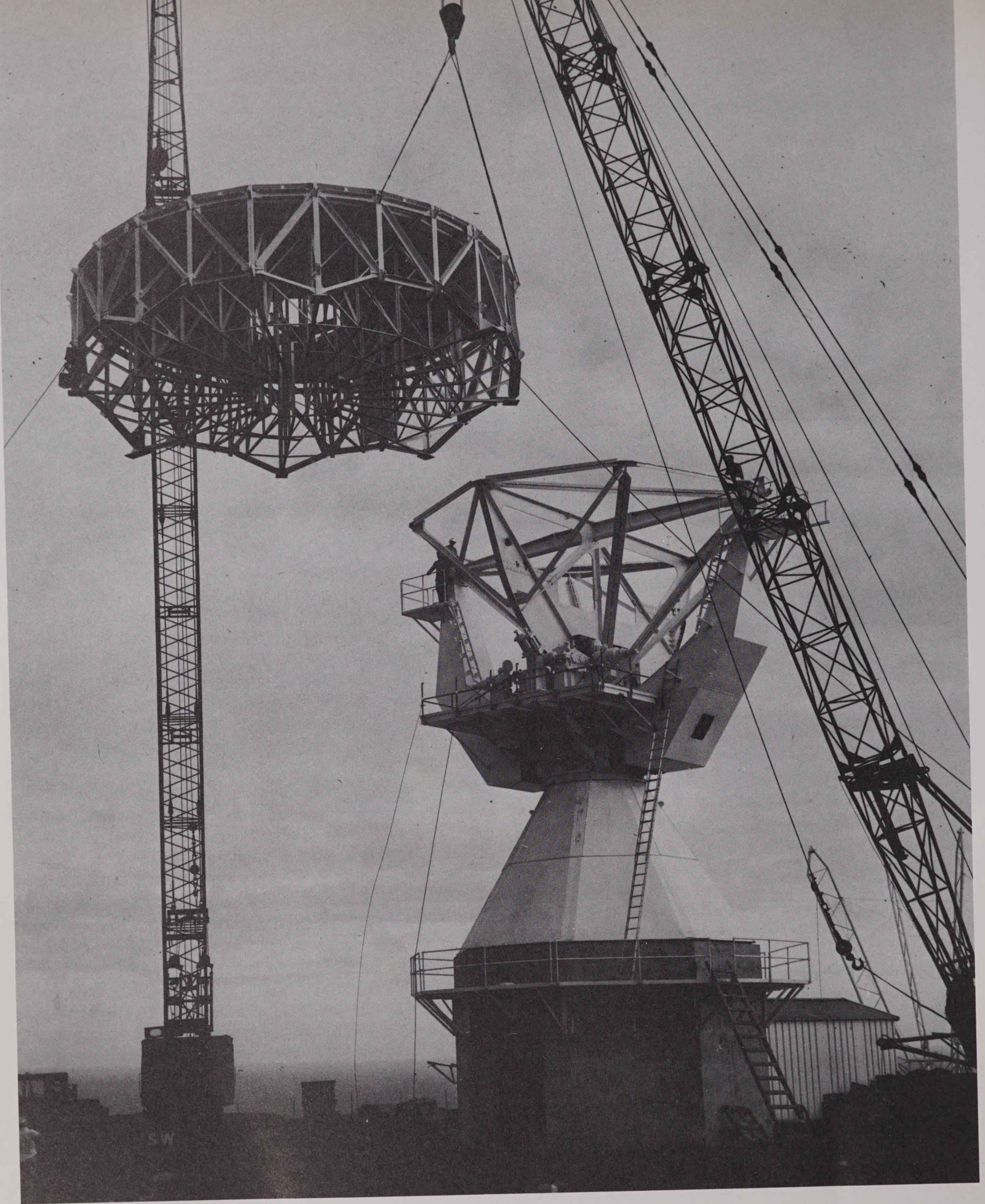
An antenna reflector is assembled at Paumalu, Hawaii. When complete, the station will be a key link in a satellite communications system serving the Pacific area.
