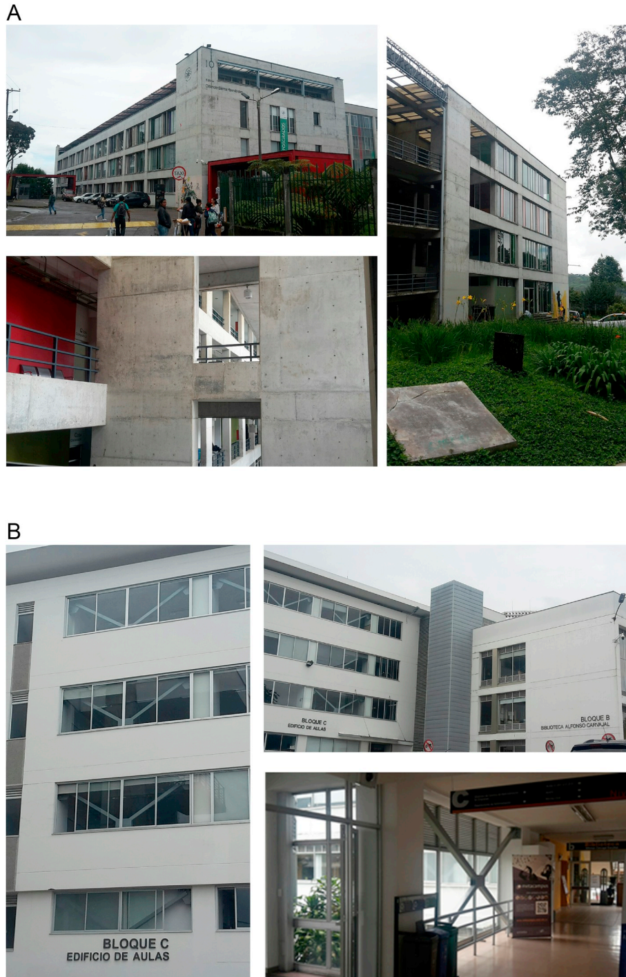
Fig. 8. (A) Seismic retrofitting of University of Caldas and National University buildings.(B) More views of seismic retrofitting of University of Caldas and National University buildings.
