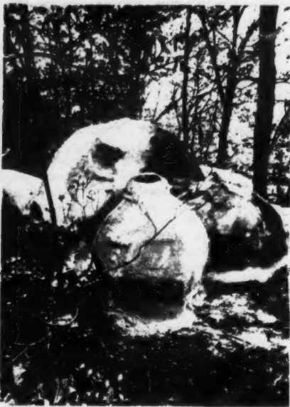
Igloo-like houses of urethane foam are formed by spraying over fabric and cable forms. Dwellings of almost any size or shape can be built in a matter of minutes.
