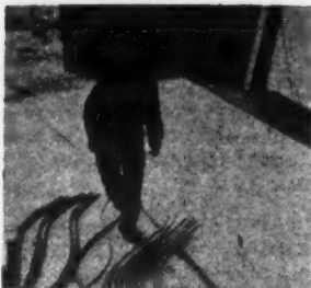
Bending the pipe frames is the first step in building a ferro cement boat, from page 48 of
