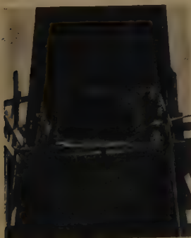
Fig. 289 An opening notch is first blasted in the 14' x 14' base of a 127-foot brick stack.
