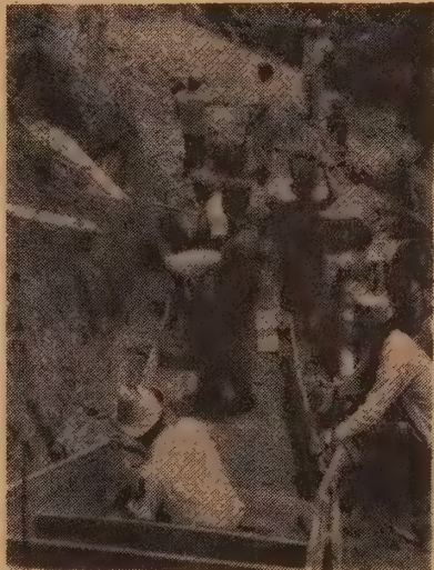
Men and children of a hillside barrio in Caracas cooperate, casapa style, to build much-needed stairs.
